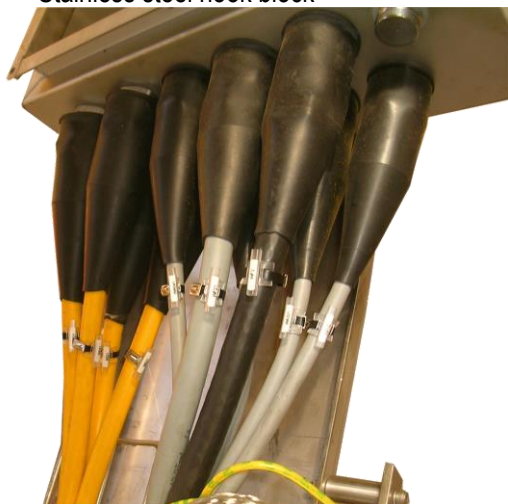
Explosion-proof electric connections
